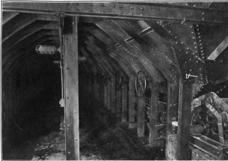
Fig. 8.—View on Tank Top under Hoppers Looking Forward, Showing After End of Starboard Conveyor
